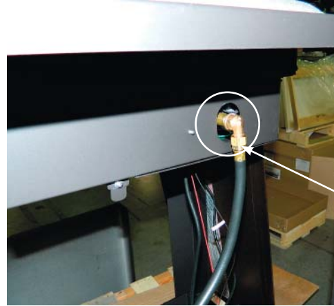
Gas connection @ unit
