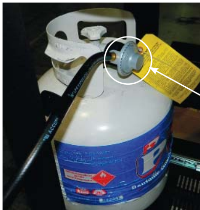
Gas connection @ tank
